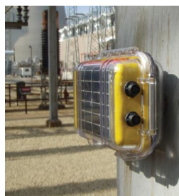
Transformer Tank-Top Temperature Sensor
